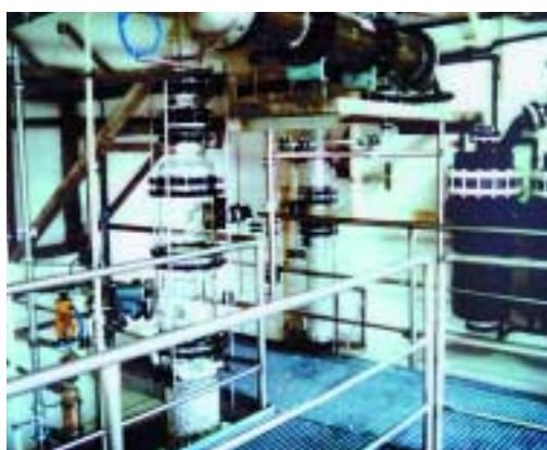
Figure 6: Third floor of the production plant giving sight into one of three separated production rooms. Upper part of the distilling column with condenser.
